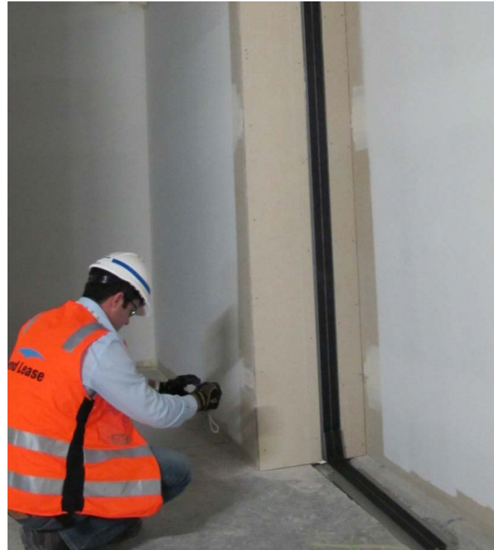
Pictured above: The MDS expansion joint cover being installed at the GCUH in the CSD area, creating a continuous joint seal across floor, wall and ceiling with 50mm cove sections.
